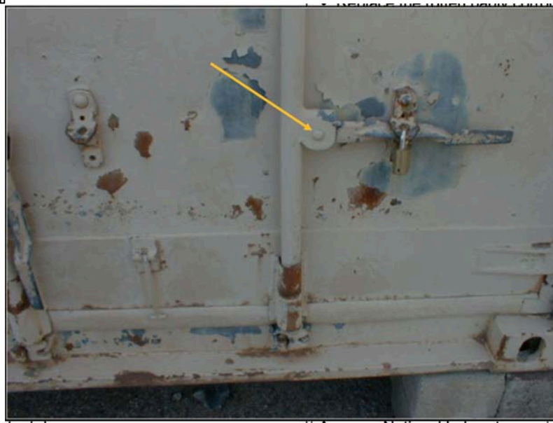
Figure 19 - Transportainer showing a lock on the handle. The arrow points to the handle's rivet that is a source of vulnerabilities for cargo theft.
